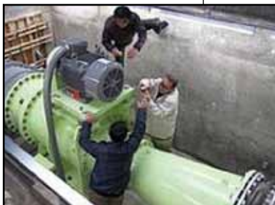
Upgrading to high efficiency motors in combination with adding biodigesters or other renewable energy technologies can save communities thousands of dollars in electricity expenses.
